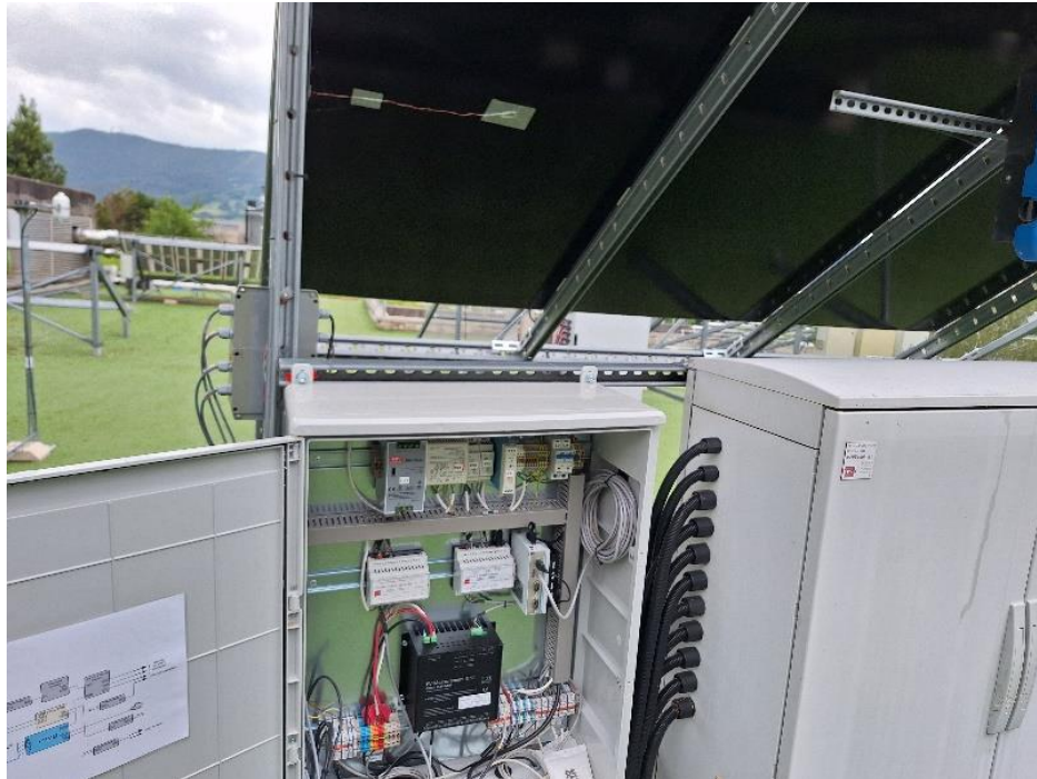
Figure 5.6: LPV-MS1X16 monitoring system
