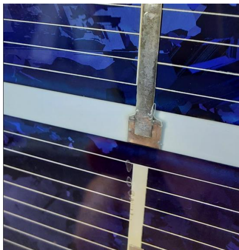
Figure 5.25: Oxidated welds in the interconnection strips of Photowatt PV module
