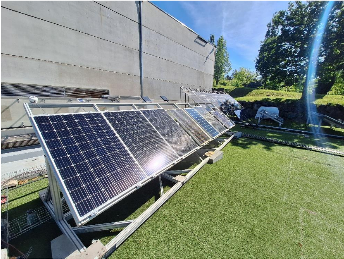
Figure 5.2: Monitoring platform oriented to the South
