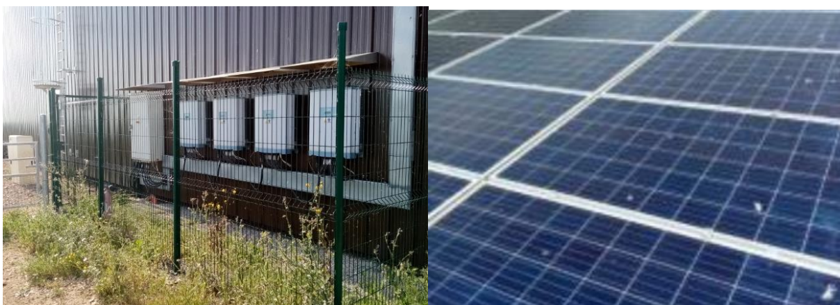
Figure 5.3: SANT PV Plant inverters and module soiling
