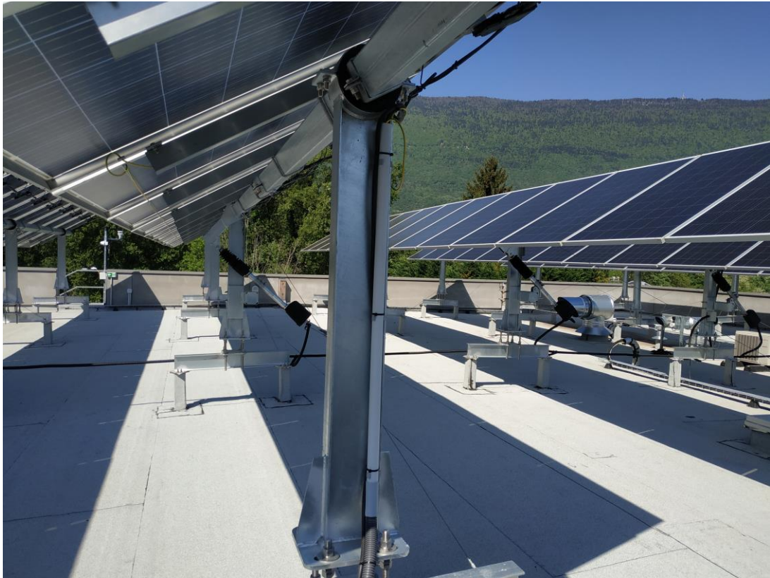
Figure 7.2: PV modules on trackers (roof part of the Cythelia installation)
